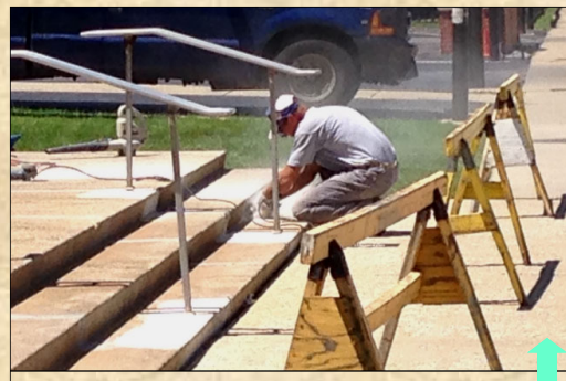
Many parishioners might have noticed the cracks in the stairs near Addison St. This past week we have sealed and repaired them preparing for the upcoming Winter season.
